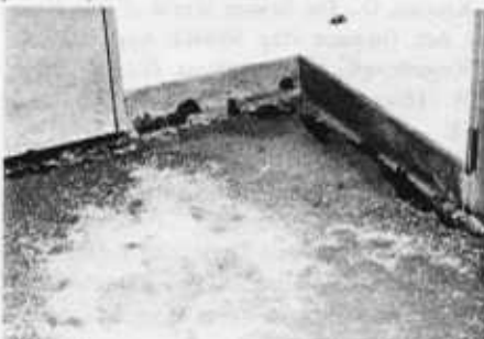
Fig. 8: Damage to areas of confinement. Epoxy paint was removed from the kennel floor by constant clawing during several months of confinement by a pit bull. Metal doors and hardware were also damaged. Dogs should not be separated by only a single woven wire fence since they will attempt to fight through the fence or pull on limbs of other kennel dogs.
